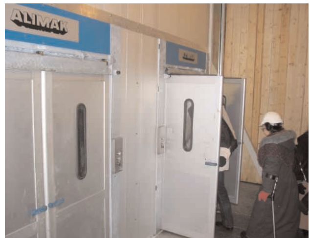
The lifts ensure anyone with a physical impairment can also enjoy the descent into the depths of the mine to explore.
