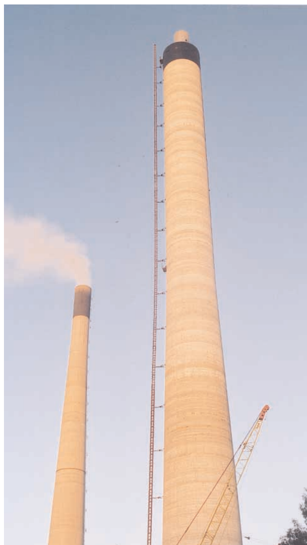
The Alimak lift is used for general inspection inside the 220 m chimney stack at the Callide Power Station, Australia
